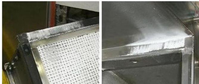
Fig. 3. Photographs illustrating seal leakage due to improper filter installation.
