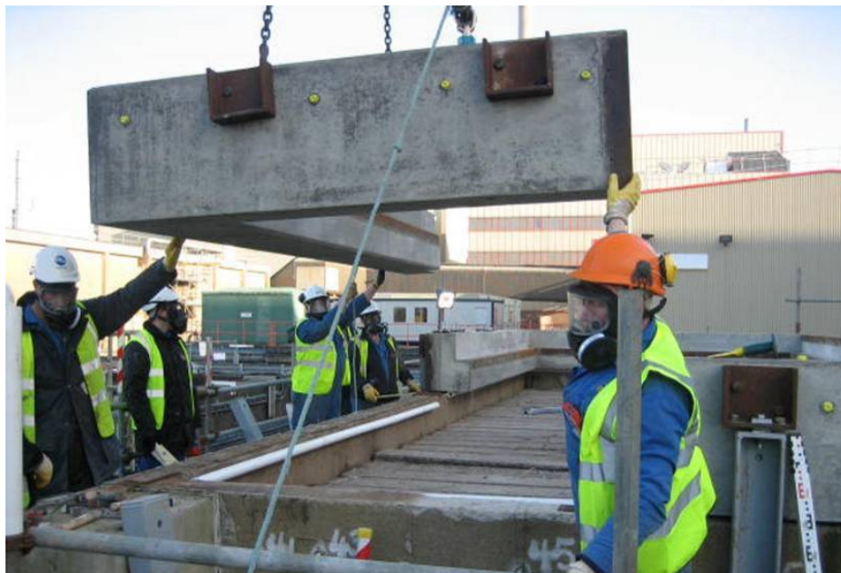
Fig. 4. Installation of ring beams to the top of the concrete cells as part of the improvements to the cell containment structure.
