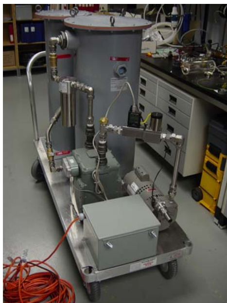
Fig.4. Dual bed air scrubbing system
