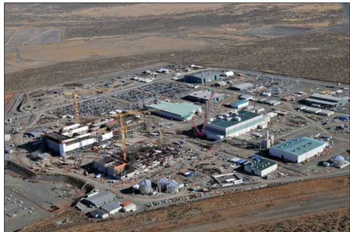
Fig. 2. An aerial view shows the immense footprint of Hanford’s Waste Treatment Plant construction site.
