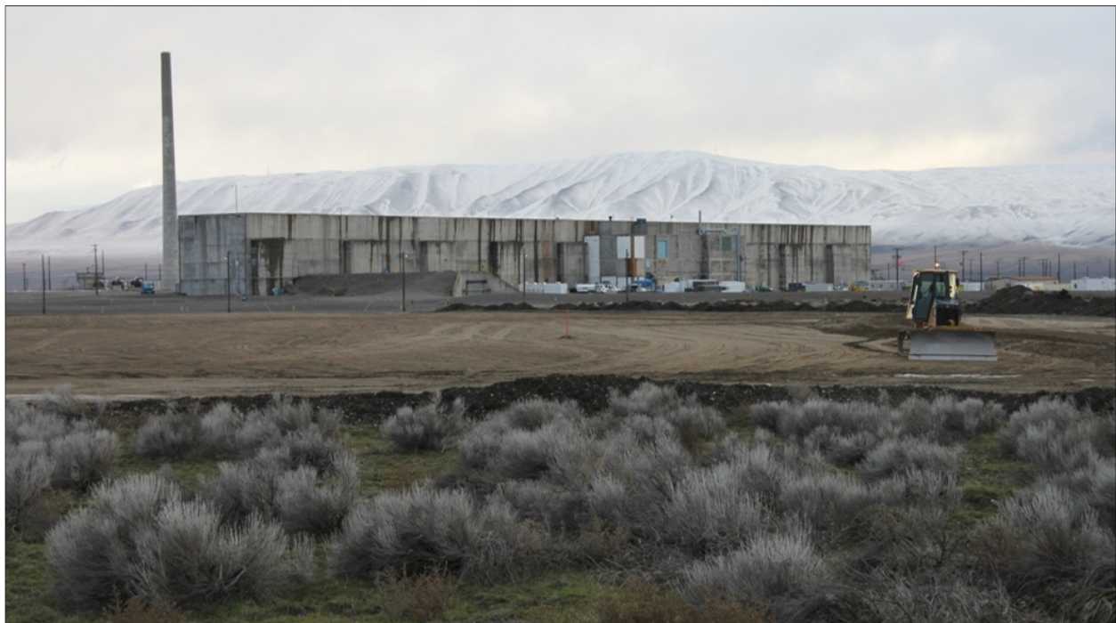
Fig. 1: The 221-U Canyon Facility at the Hanford Site, as CH2M HILL D&D workers prepare the site for placement of fill for the canyon's eventual demolition.
