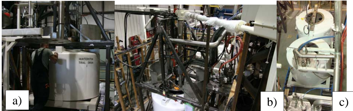
Fig 4: CILWPP FAT Photographs a) 3m 3 RMWD drum b) Filling Station c) Capping Grout and Lidding Stations
