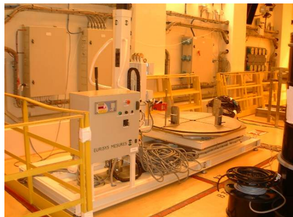
Figure 4 – Drum Screening Station
