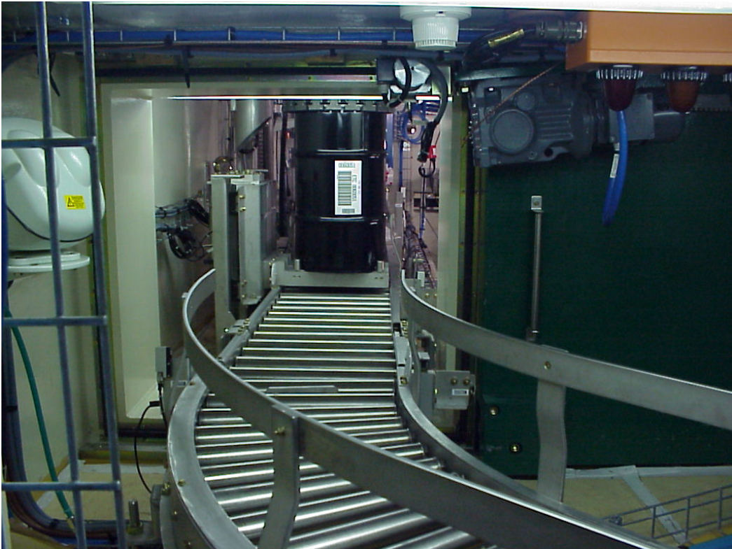
Figure 3 – Drum Transfer System
