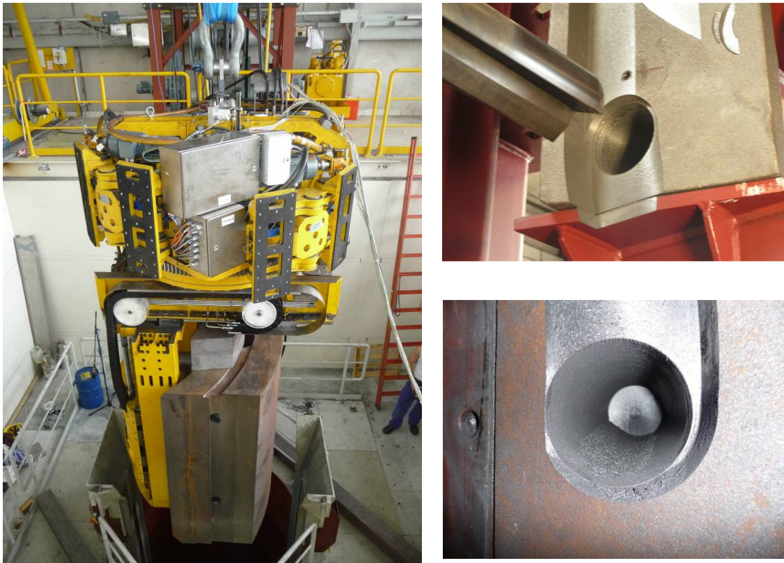
Fig. 3: Drilling and lifting up of the primary shielding segment in the mock-up
