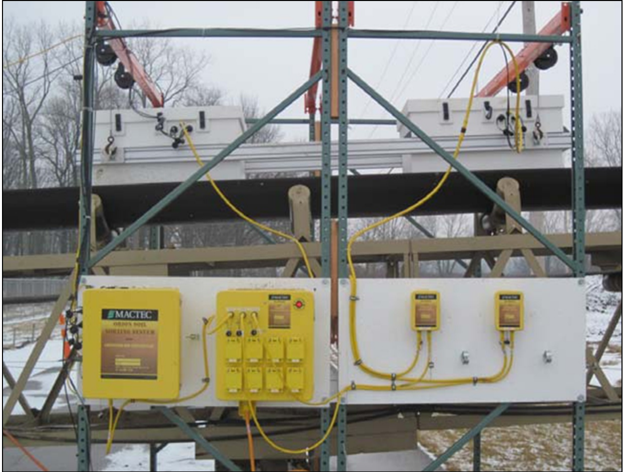
Figure 4 Auxiliary QA/QC Detection System Mounted on Conveyor #6
