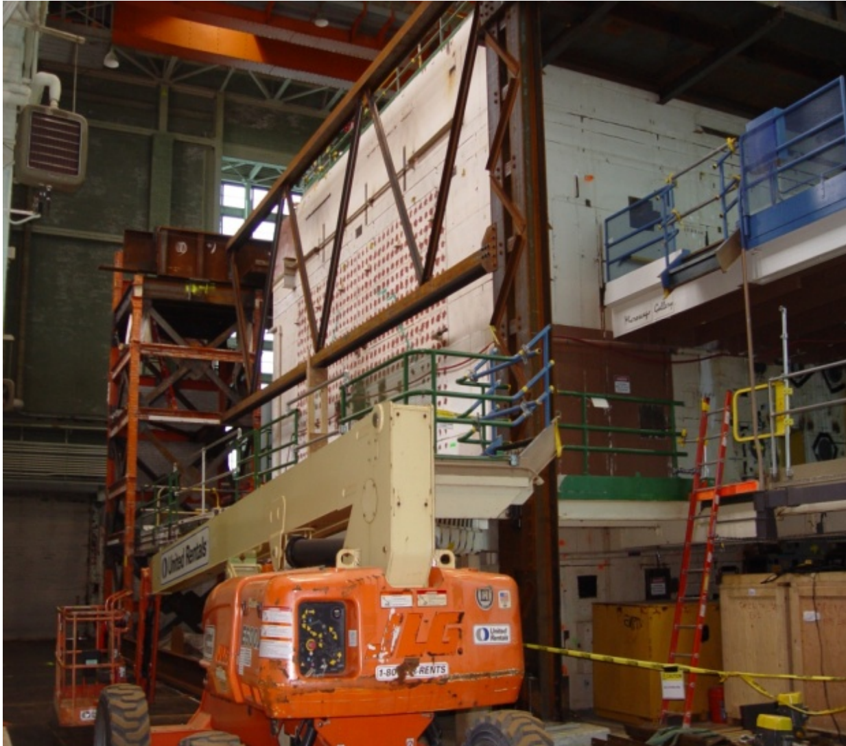
Fig. 3. Structural steel system – North face column with converted elevator shaft tied together with truss number 2
