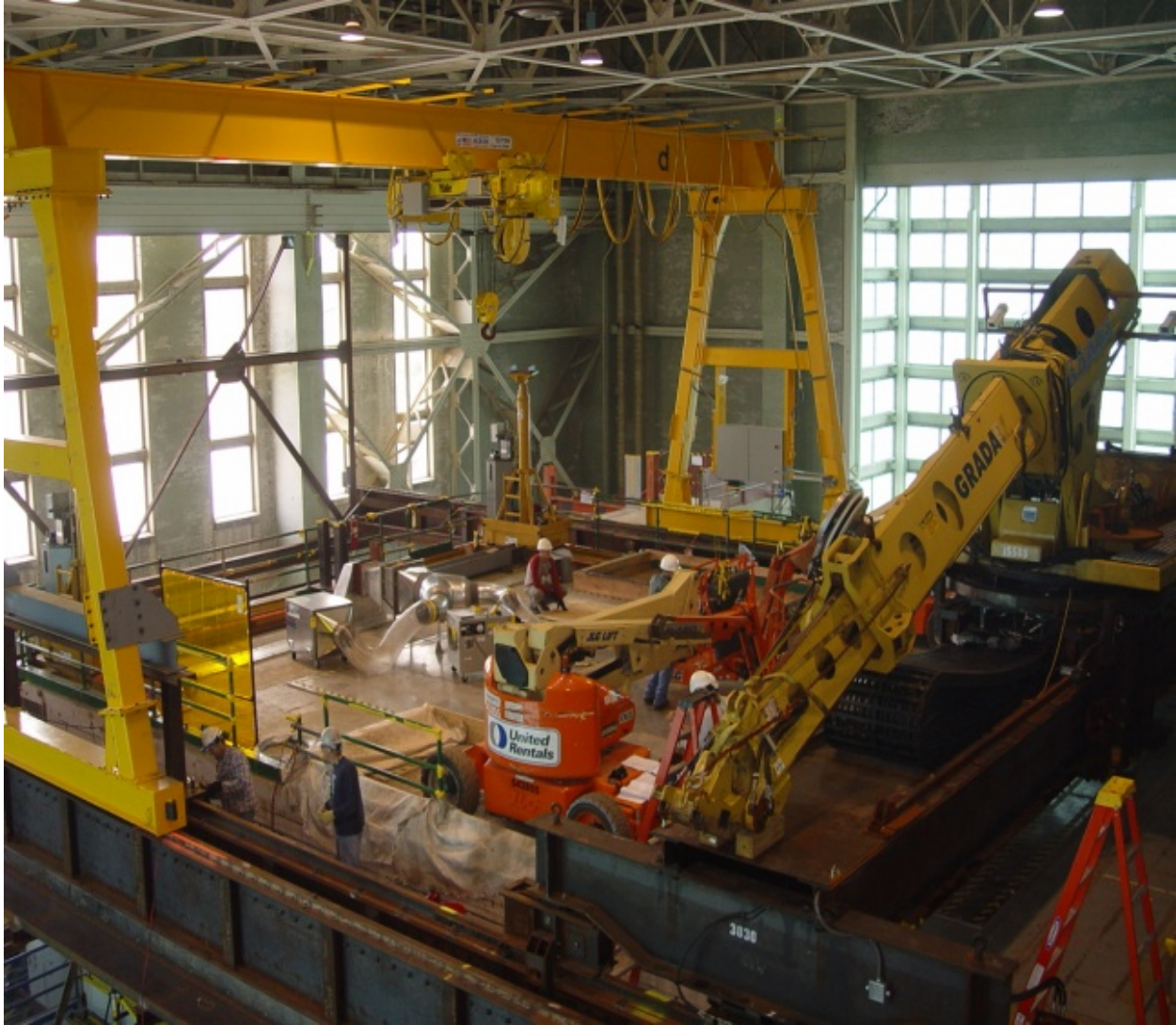
Fig 2. Reactor top straddled by remote gantry-mounted excavator & support crane on an independent rail
