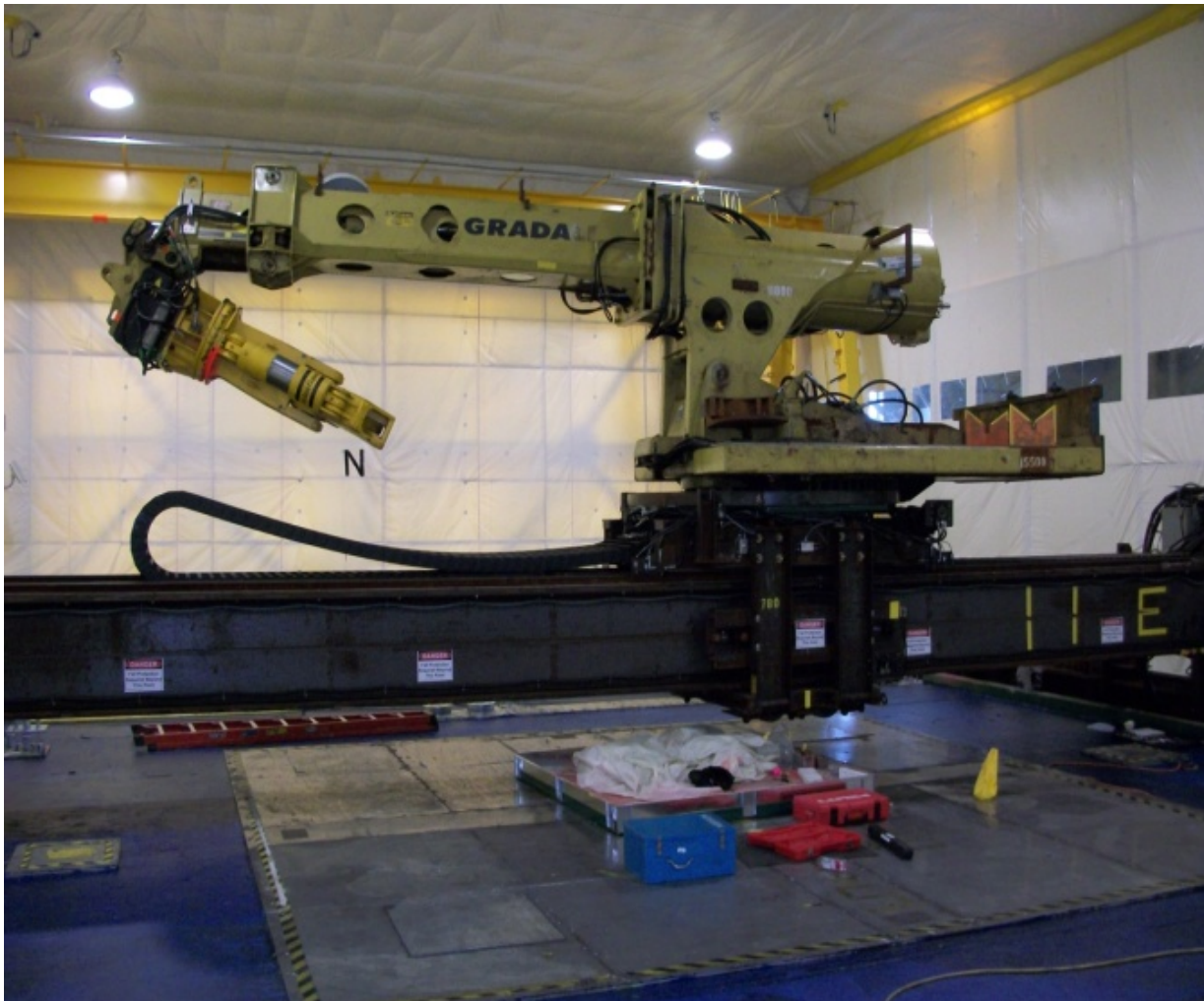
Fig. 1. The excavator with the shear attachment is shown here above the access plugs inside the contamination control enclosure (containment).
