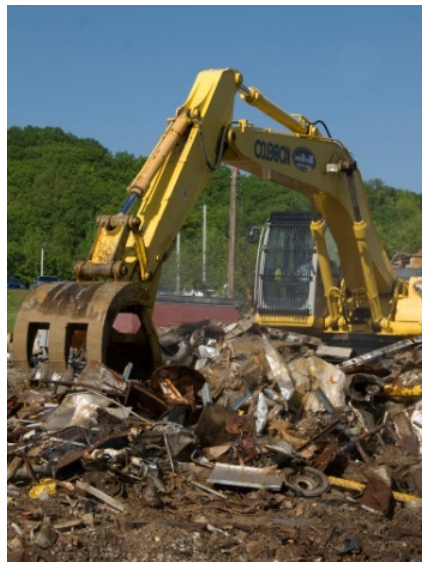
Figure 7. Heavy Equipment moves scrap metal during characterization to access sampling points within OSY pile
