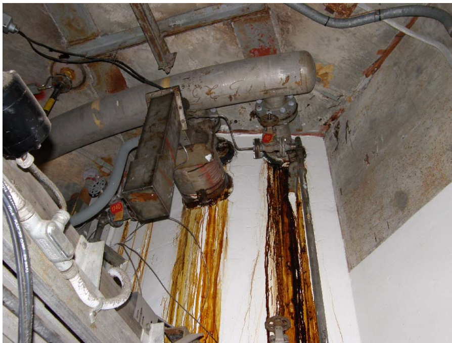
Figure 1. This photograph was taken in building 105-L at the -20 elevation. It shows degraded polyurethane sealant leaking from piping penetrations in the reactor biological shield wall and the painted surfaces that the sealant contacted.
