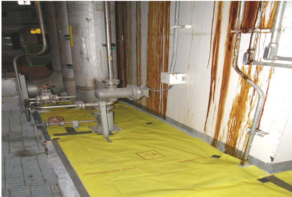
Figure 4. This photograph was taken in building 105-L at the -40 elevation near the Reactor Pin Room where the horizontal surfaces have been cleaned by scraping, covered and labeled.
