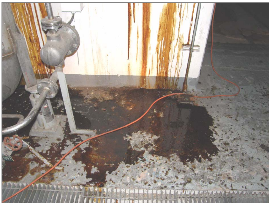
Figure 2. This photograph was taken in building 105-L at the -40 Elevation adjacent to the Near Side Pin Room Entrance. It shows deteriorated sealant which has seeped to the floor next to open grating. Beneath the grating is a trench that ultimately provides a pathway to building sumps.
