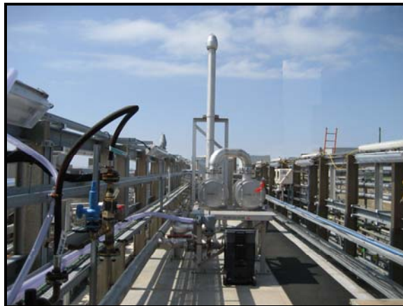
Fig 5 - Installation and commissioning of the Passive Off Gas System for the Pile Fuel Cladding Silo.
