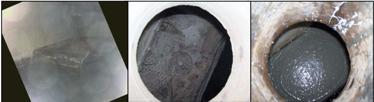
Fig 2 –Image of Weirbox inside wet bay, showing its position relative to the waterline and top view of weirbox prior to and post isolation.
