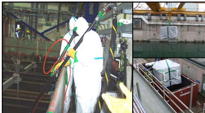
Fig 4 - Water jet lancing in the Decanning bays and removal of skips from main pond
