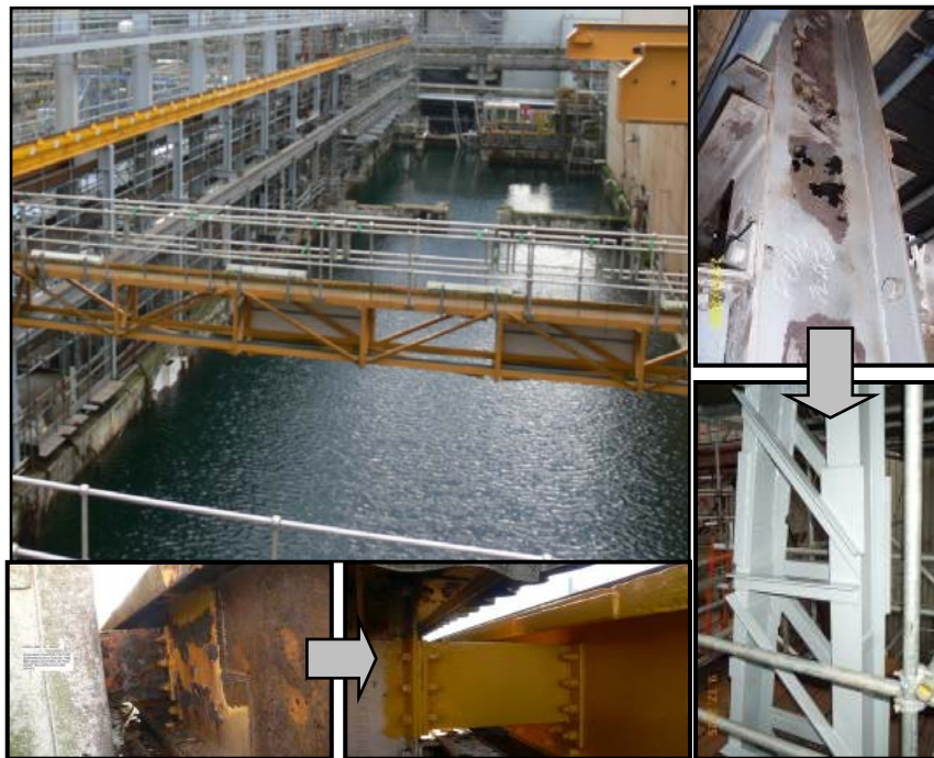
Fig 3 – Position and condition of the Gantry Structure
