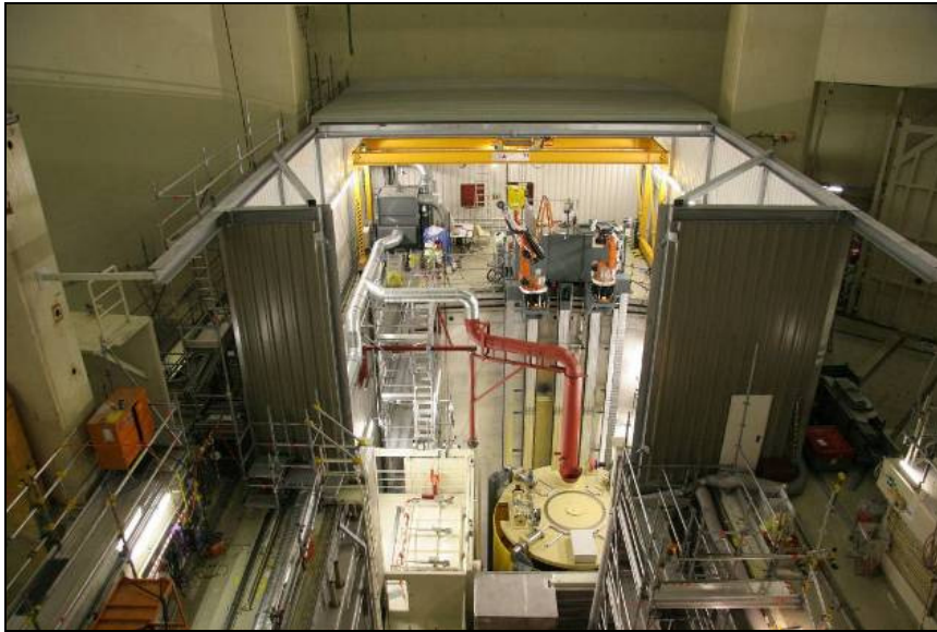
Fig. 2. Total view over the spent fuel pool with dismantling and packaging facilities
