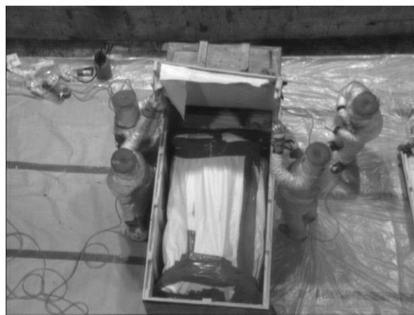
Exposure of ductwork in plywood box
