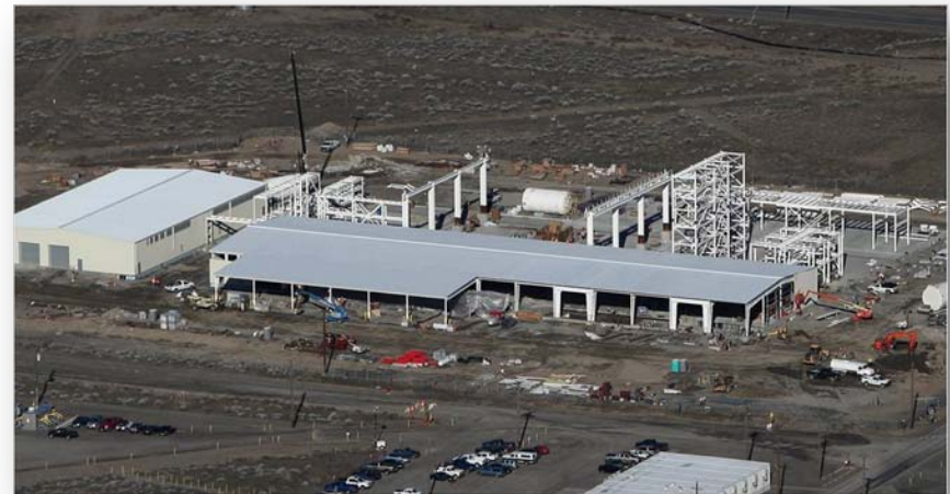
200 West Groundwater Treatment Facility
