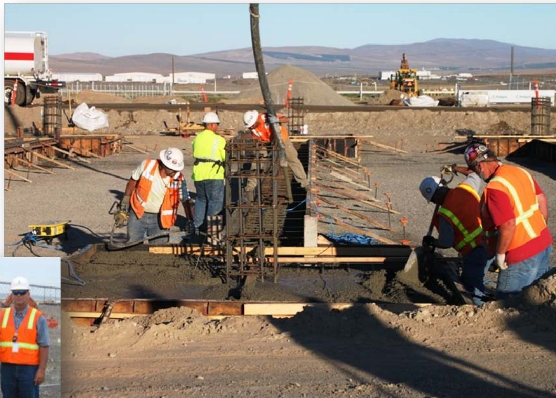
Workers Place Concrete Footings for the 200 West Pump and Treat Rad. Building
