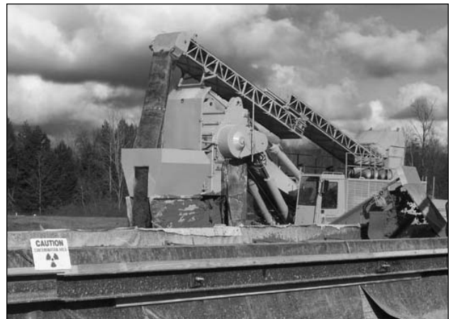
A "one-pass trencher" was used to install a permeable treatment wall to capture Strontium-90 from a groundwater plume.
