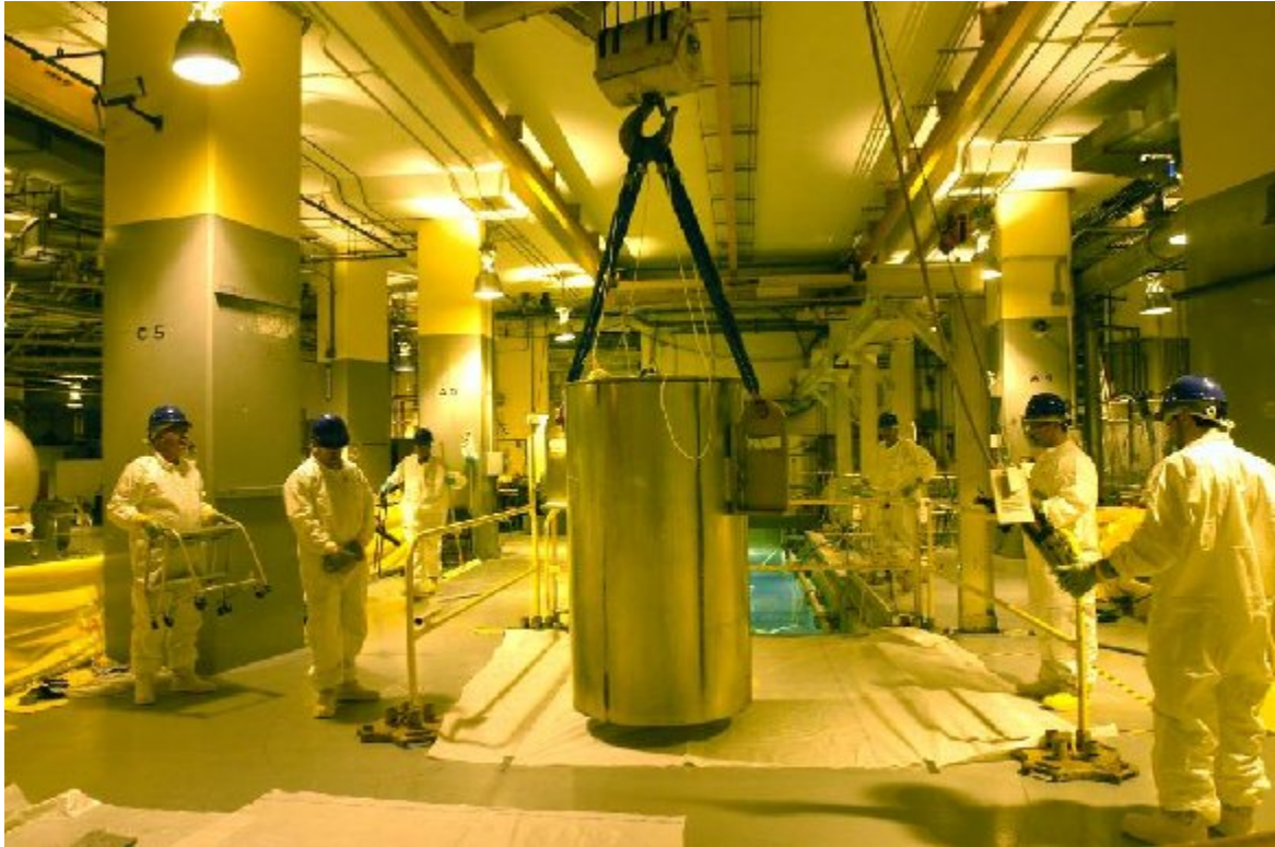
Getting ready to place CNS 1-13G cask into spent fuel pool to load control rod blades underwater.
