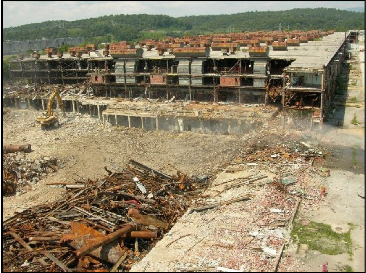
Fig. 4. Demolition of the West Leg exposes a cross-section of the K-25 Building. From bottom: vault, enrichment-cell level, pipe gallery and operating floor. (Photo courtesy of BJC)
