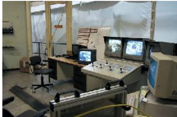
Fig. 10: Remote operation console in the control room
