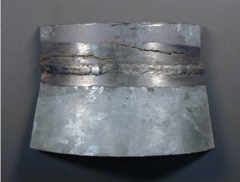
Figure 2. Section of ventilation ductwork removed from the exhaust of the purge ventilation system. Two cracks are evident. A third crack, located on the opposite side of the weld, occurred on the inside surface but did not penetrate to the exterior. Magnification is 1.25 X.
