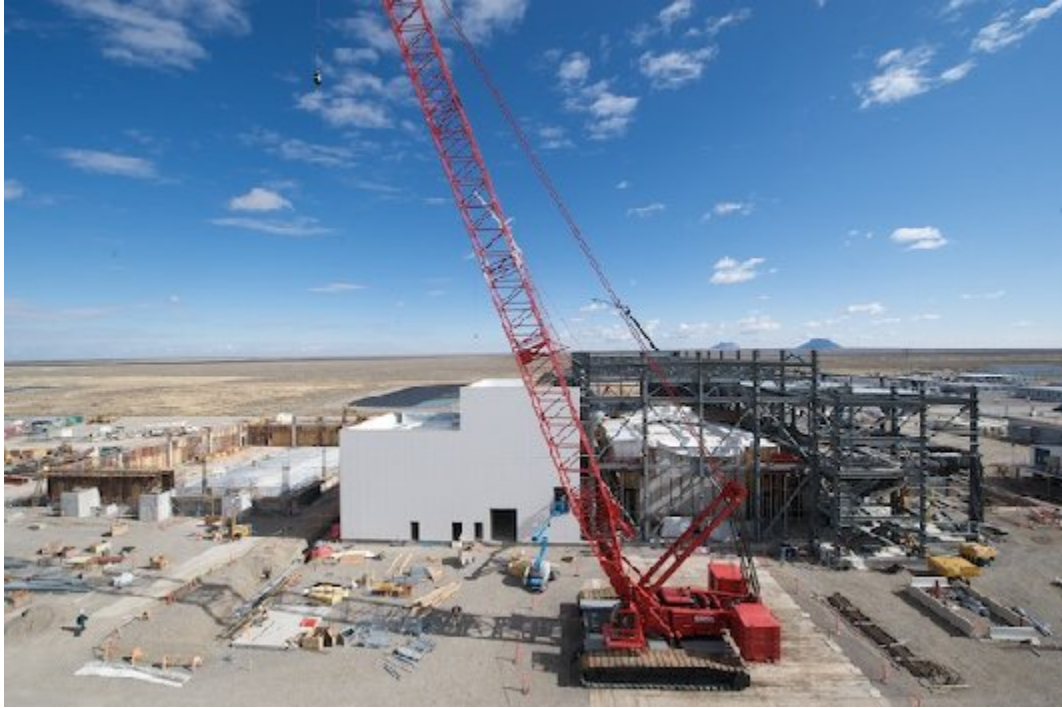
Figure 1. IWTU treatment building and product storage building under construction in the fall of 2009.
