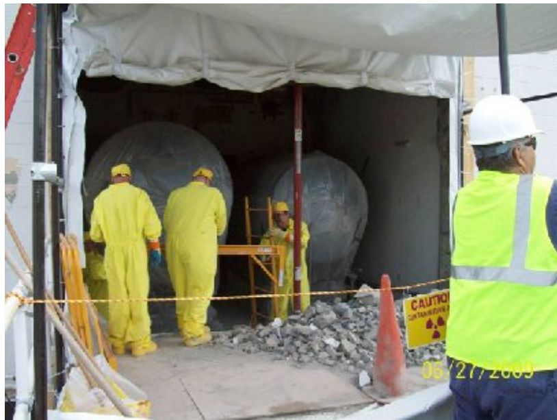
Fig. 2. The two vessels in the Hot Acid Cell are exposed through the opening cut in the wall of the cell as the vessels are prepared for removal through the cell wall.
