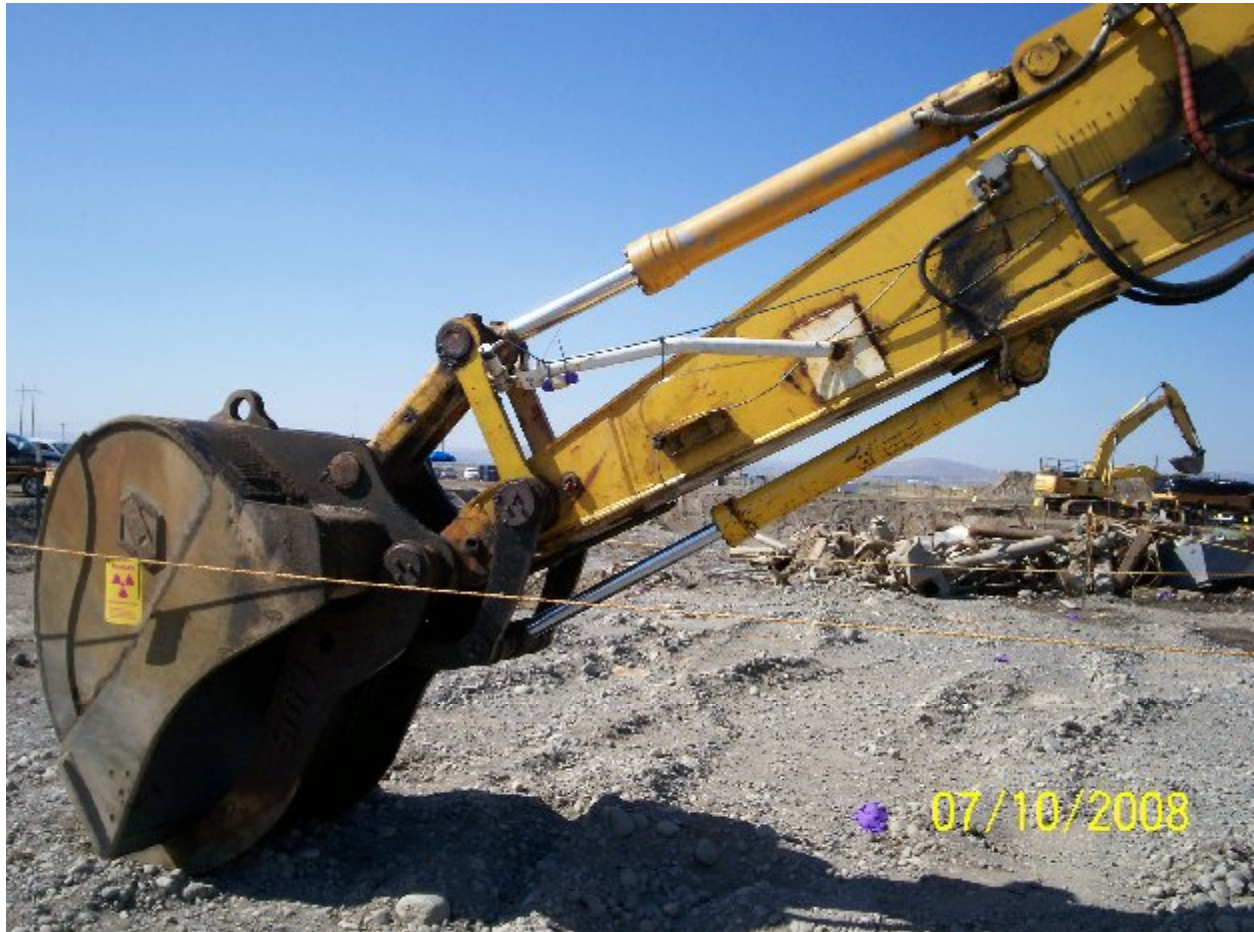
Fig. 2. Excavator bucket and arm showing infrared thermometer and radiation meter mounted on end of white metal pole and photoionization detector intake tube running along length of arm.
