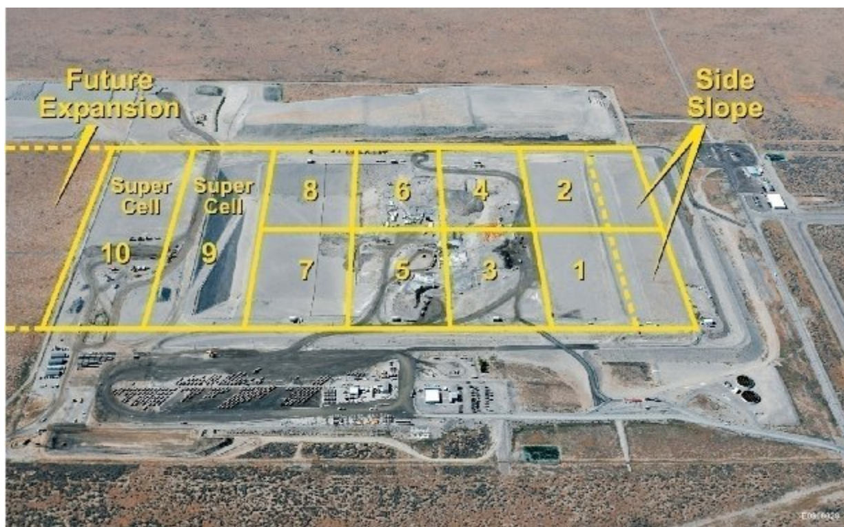
Figure 1. Construction of super cells 9 and 10, which is underway at the U.S. Department of Energy's Environmental Restoration Disposal Facility, will expand capacity by 50 percent. The $55 million expansion and another $45 million in upgrades are funded by the American Recovery and Reinvestment Act.
