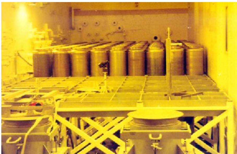
Fig. 1. 275 HLW canisters are currently safely stored in the Main Plant Process Building.
