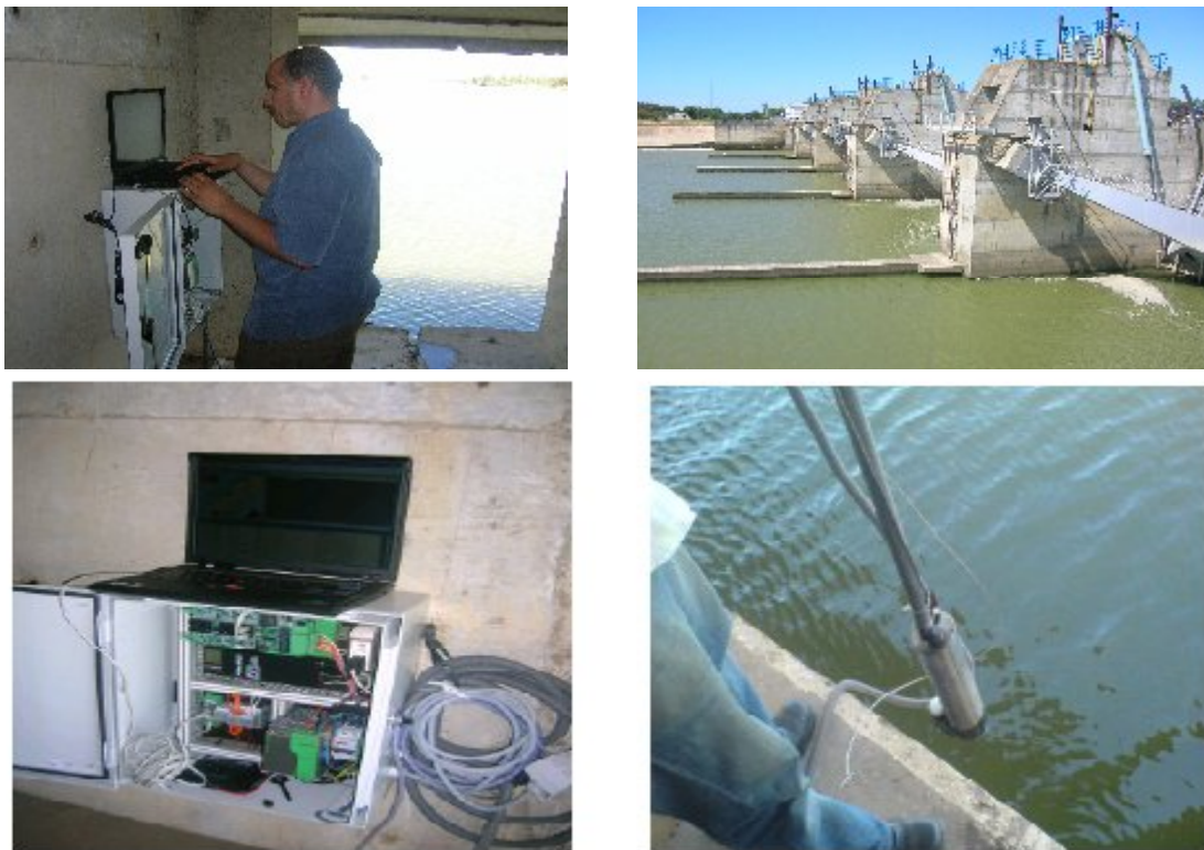
Fig. 4: Probe installed in Sebou river (Barrage de Garde)
