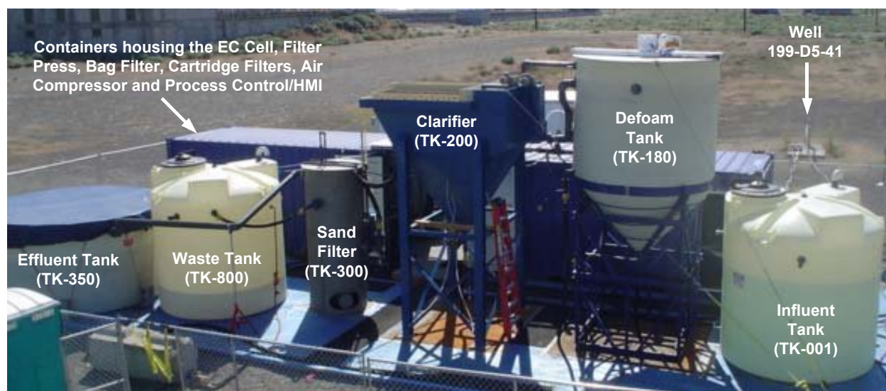
Figure 3. Overview Photo of the Installed Electrocoagulation Treatability Test System.
