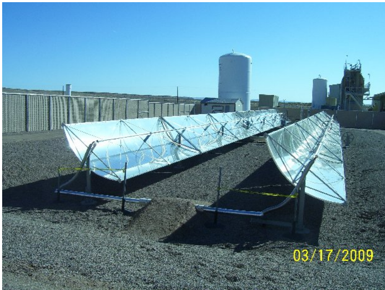
Fig. 4. Tuba City, Arizona, Solar Hot Water Heating System
