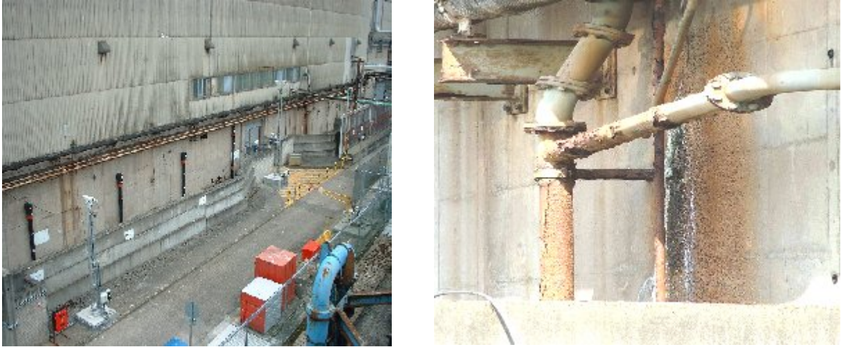
Fig 3 showing the service lines above the purge pipes and a close up of an example of a corroded section of the purge pipes
