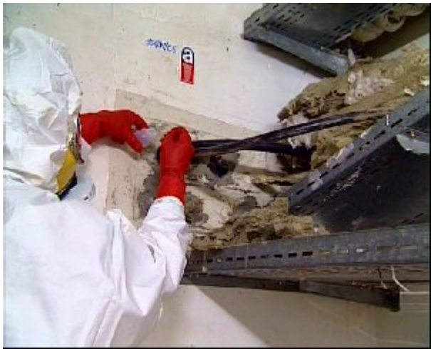
Fig. 4. Asbestos-containing Feedthroughs, Sampling
