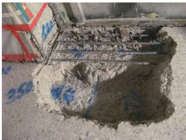
Fig. 6. Removed Hot Spot
