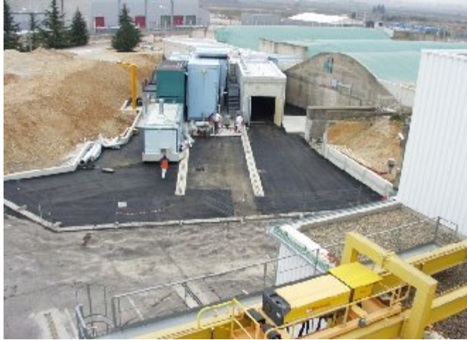
Figure 1 :ERC Installation (Marcoule Site)
