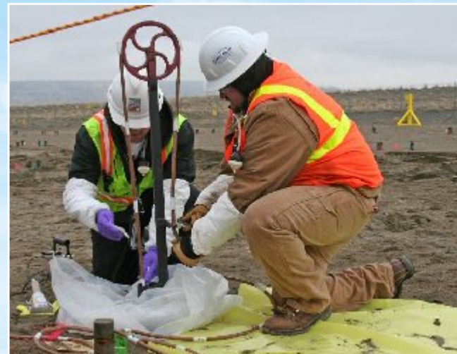
Workers drop a multi-detector probe down a cone penetrometer to measure radiation activity at the 618-10 Burial Ground.
