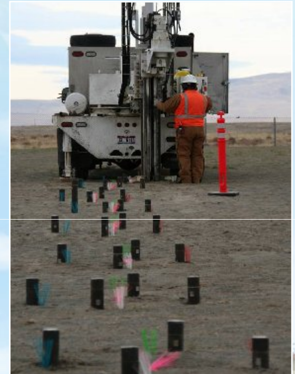
Installation of cone penetrometers around the vertical pipe units at the 618-10 Burial Ground.
