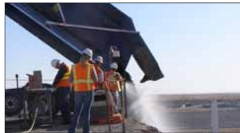
A super dump truck unloads soil at the Environmental Restoration Disposal Facility.
