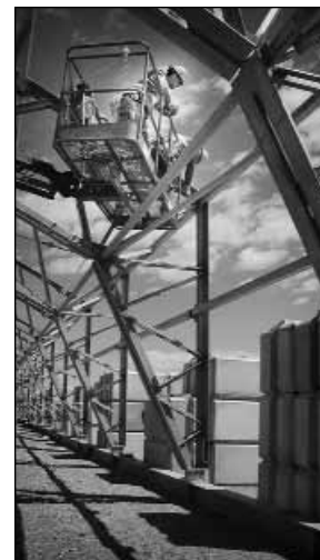
Workers prepare the steel structure of the ARP IV facility before the fabric skin is installed.
