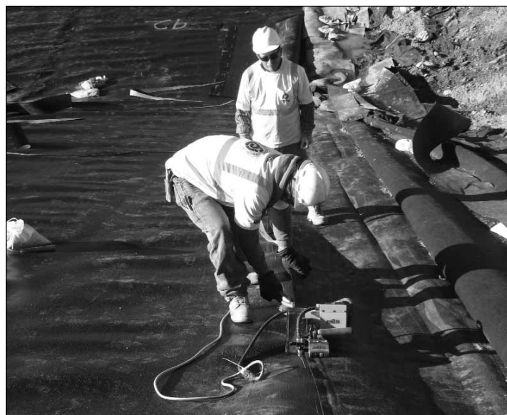
ESI workers weld the final seam in the EMWMF Cell 5 secondary geomembrane. The membrane to the right is the run-out of the Cell 4 geomembrane that was installed in 2004. The membrane to the left is the new secondary geomembrane for Cell 5. The wedge welder heats both sheets of membrane to 500 degrees Fahrenheit, then fuses them together in two parallel strips.
