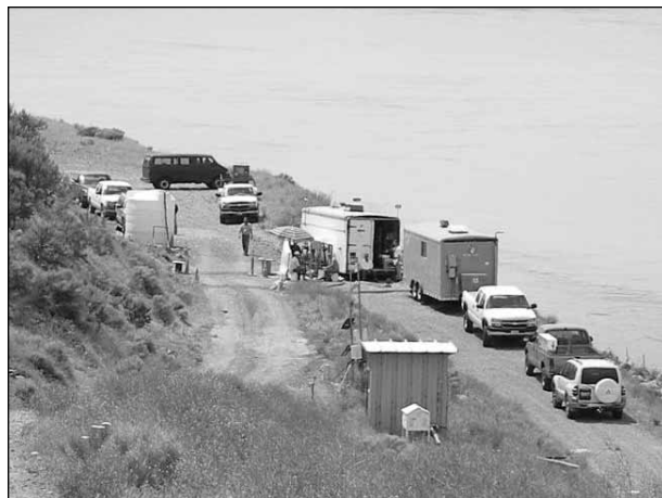
PNNL scientists install a contaminant barrier along the Columbia River shoreline on the Hanford site.
