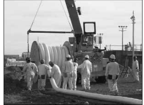
Hanford tank farm workers rolling out a Hose-in-Hose Transfer Line
