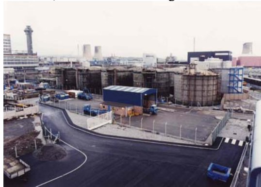
Figure 1 – Floc Storage Tanks in the early 1990s
