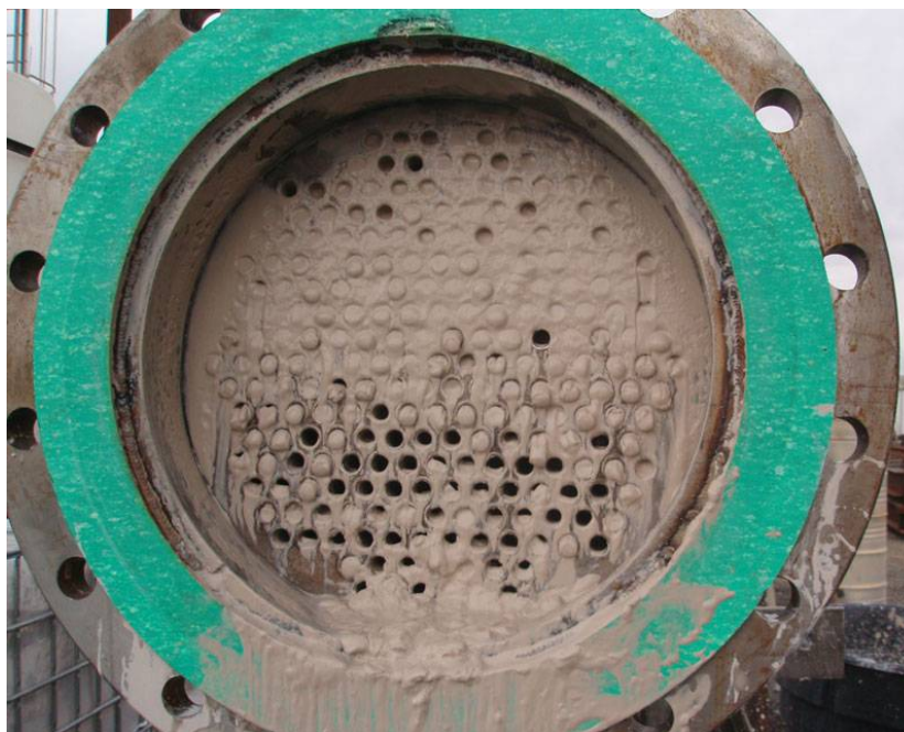
Fig. 2. Partial opening of tubes after venting of shell side of filter during Phase 1B
