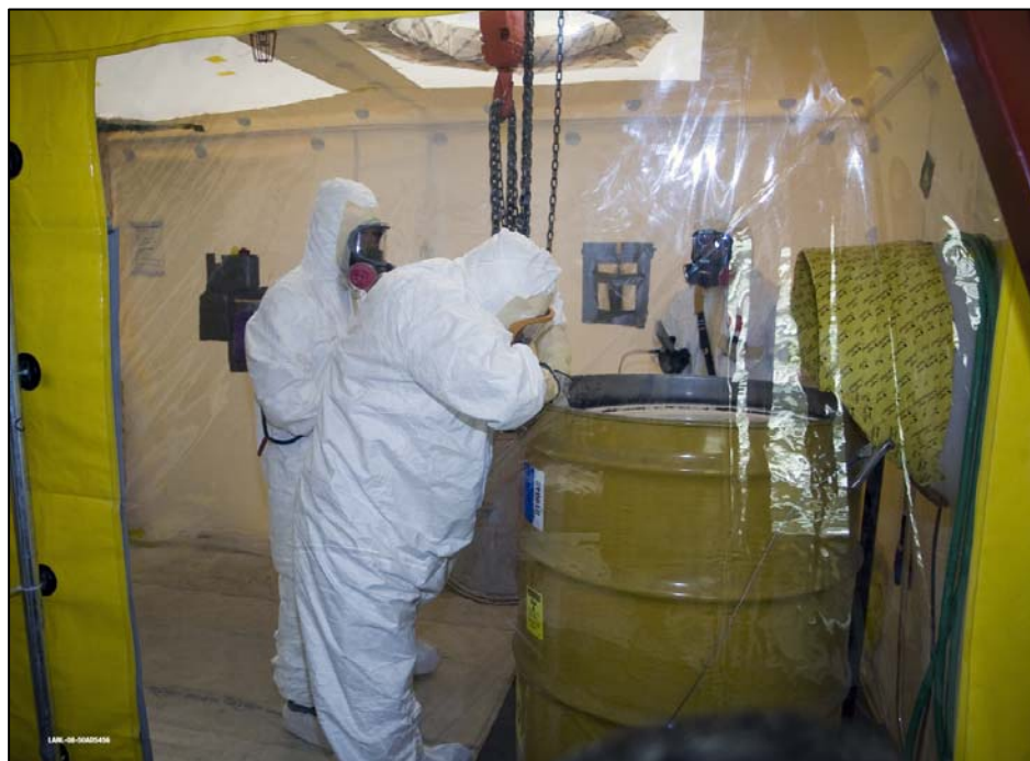
Figure 2. Special facility and equipment capability was required to vent high-activity unvented drums before repackaging.
