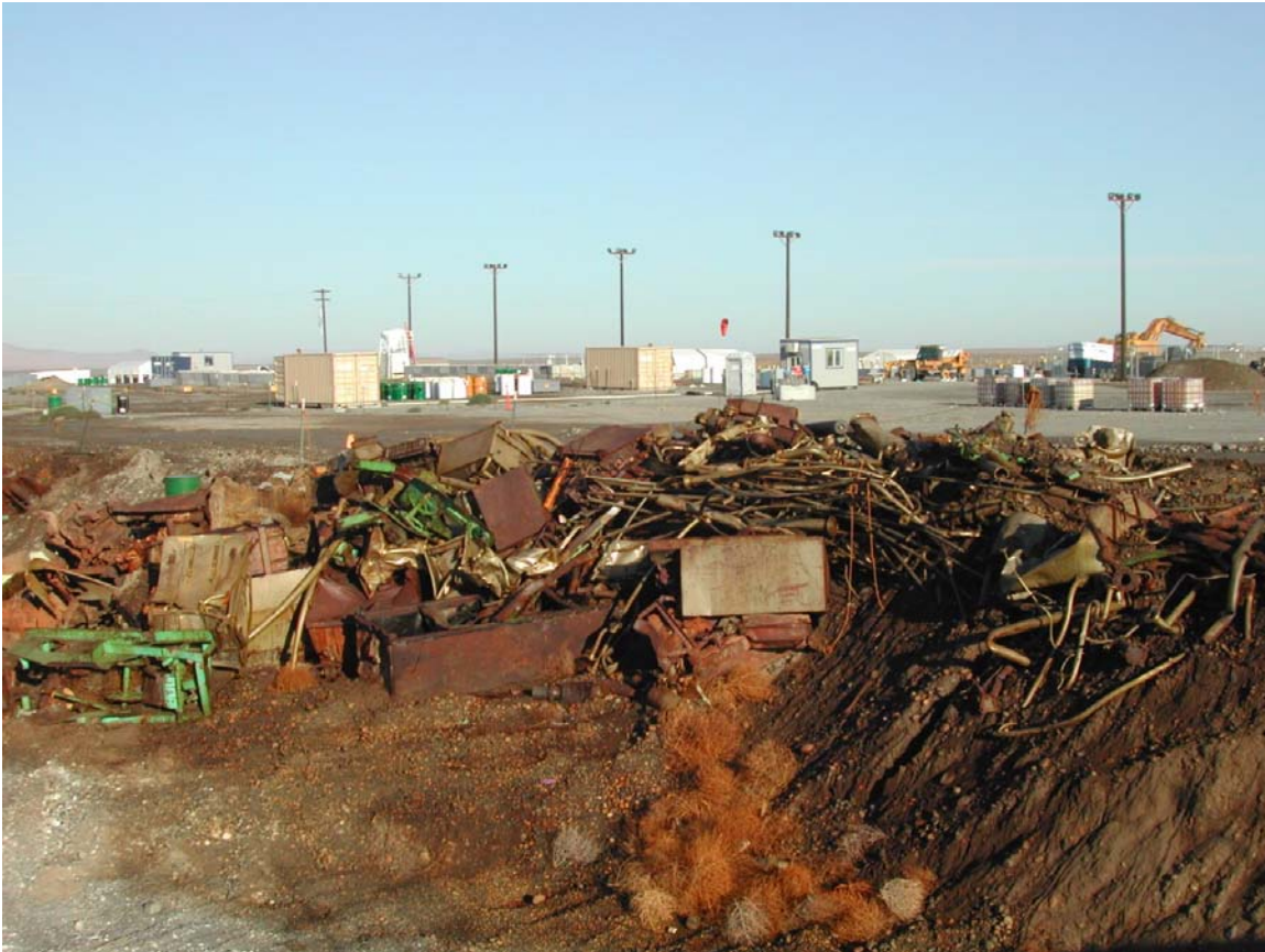
Fig. 4. Metal Debris coated with Fixative prior to shearing.
