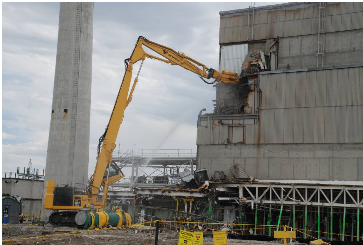
Fig. 3. A high-reach excavator was used to demolish the F-G (reactor interface area) area.
