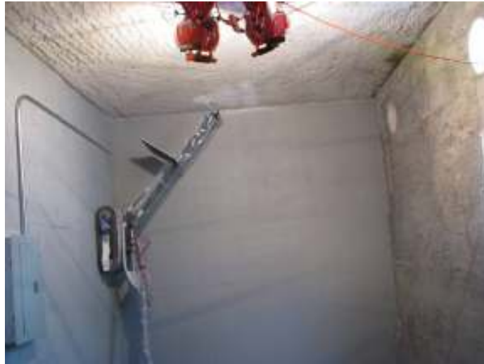
Figure 4. ICM climber beginning to apply fixative (Promar 200) to hot cell mockup ceiling
