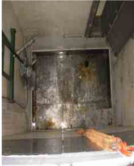
Figure 15. Spent Fuel Pool completely drained and sealed
