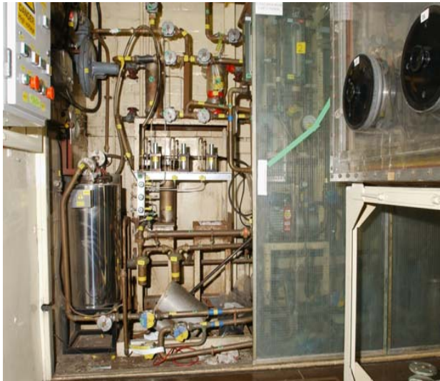
Lab 2 Argon Suite Treatment Plant
