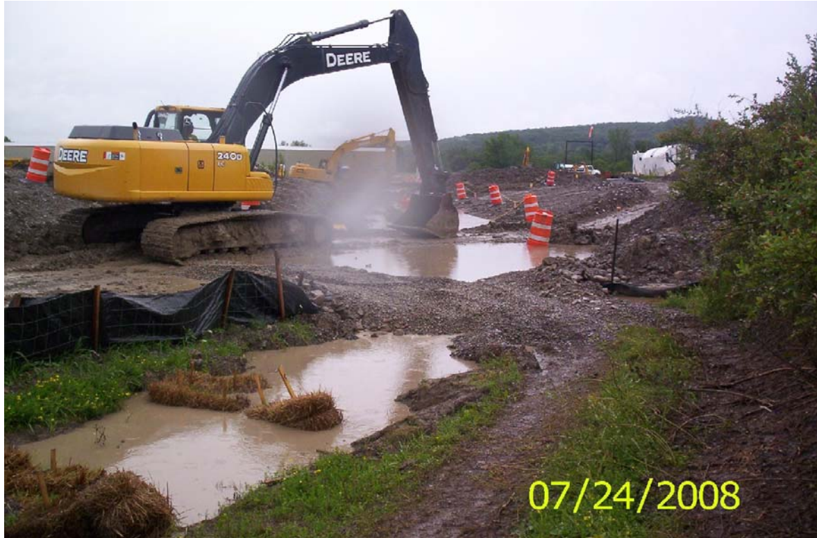
Figure 2. Stormwater pollution prevention barriers -- repairs and maintenance in progress after a heavy rainfall event.
