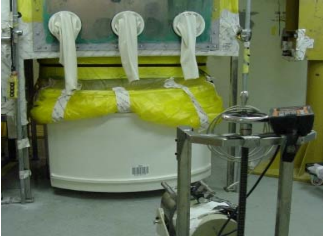
Figure 3 – Field-HRGS survey and analysis of TRU waste SWB container while still attached to an airborne HCA material reduction area and glovebox.
