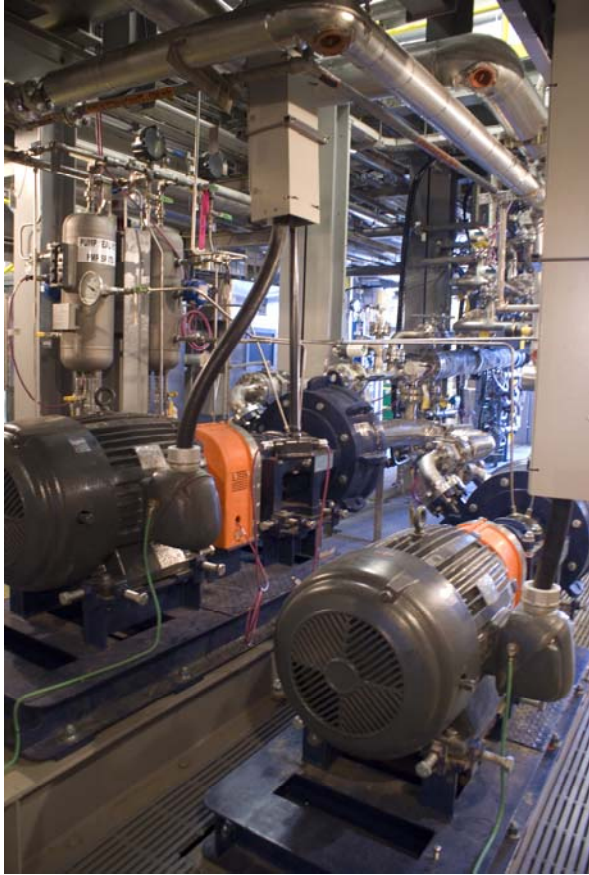
Fig. 2. Ultrafiltration Loop Pumps on the First Operating Level.
