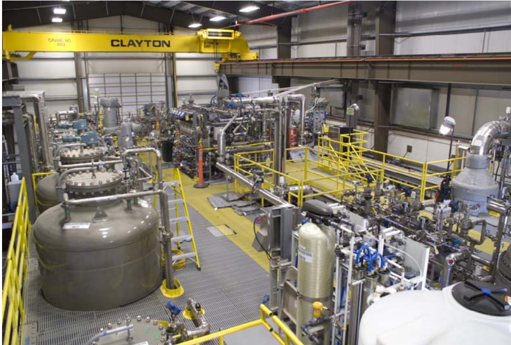
Fig. 1. Upper Operating Level of the Pretreatment Engineering Platform.
