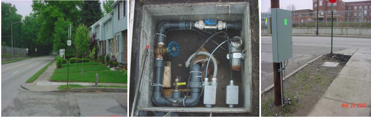
Figure 13. MW-28 MTBE Cut-off Pumping Well Photographs.
