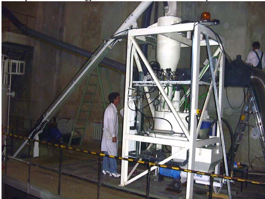
Fig. 2. Installed radioactive wastes cementation facility in reactor's hall.
