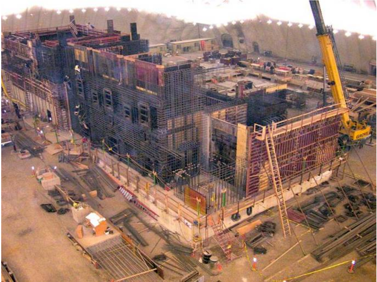
Fig. 4. An aerial view of extensive rebar during in-progress construction of the IWTU process building.
