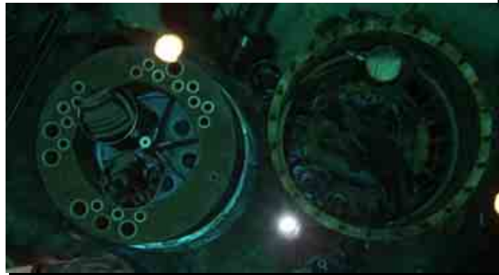
Material in HFIR pool – activated reactor components like beryllium reflector, 1M R control plates, bearings, etc.
